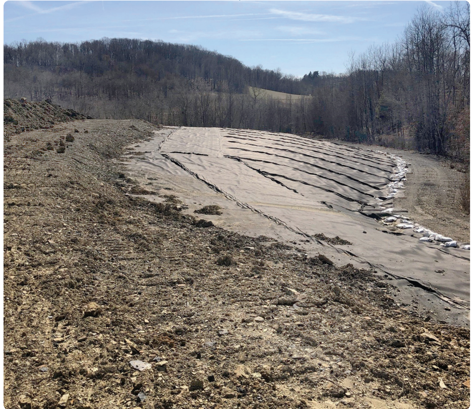
Two feet of clean cover soil is being placed over the cap on a former impoundment reclosed under an agreement with the DEP.
